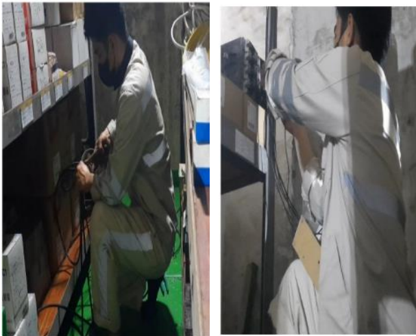
Fig. 10. The process of cutting and connecting cables on shelves in the warehouse
